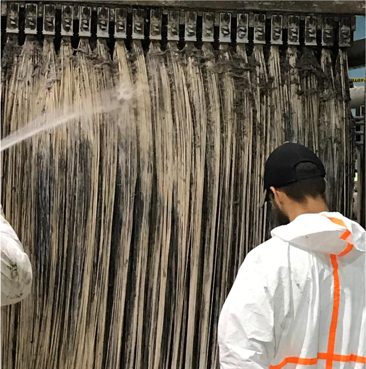
► Picture 2 – Condition of filters as cleaning starts in December 2019
